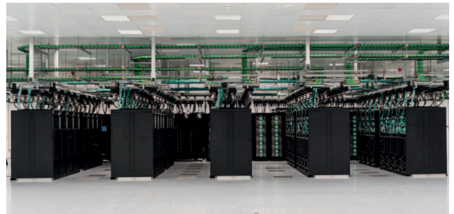
FIGURE 2 The data centre houses ECMWF's new HPCF.
