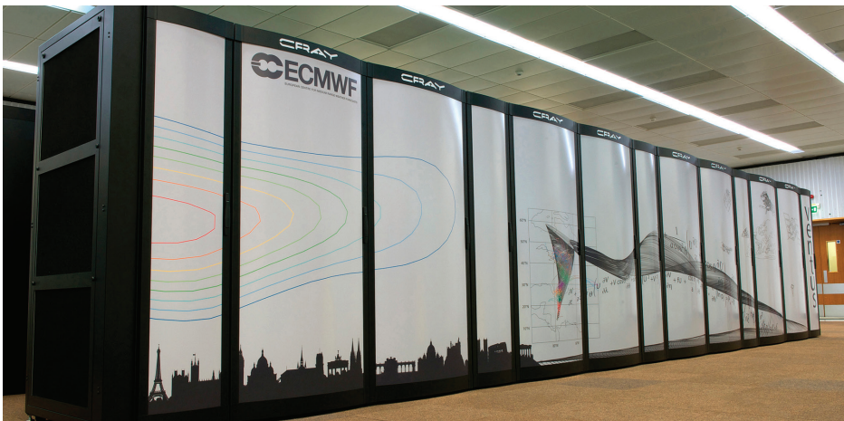
Figure 1 'Ventus' is one of the two Cray XC-30 clusters installed in ECMWF's data centre.
